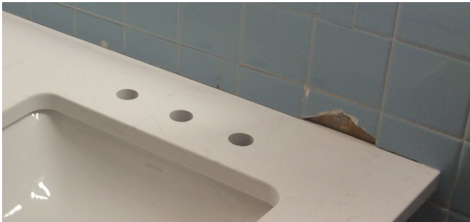
Damage to existing tile
